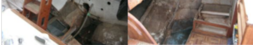
Aft Cabin area gutted
